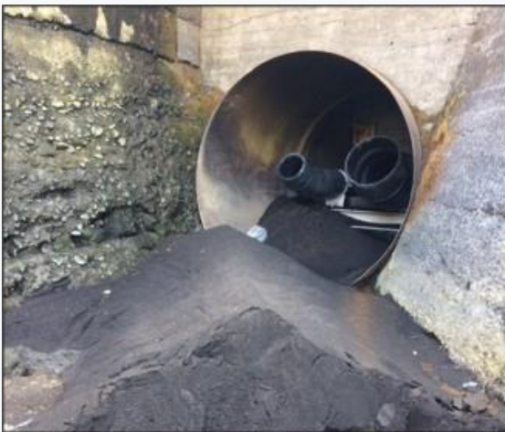
Sediment removed from the intake system
