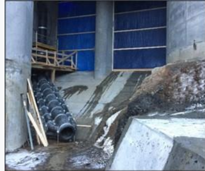
SediCon Sediment Excluder installed at the intake
