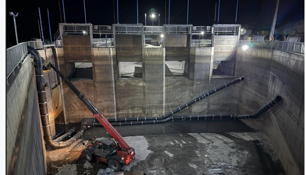
SediCon systems installed upstream of the desanders
