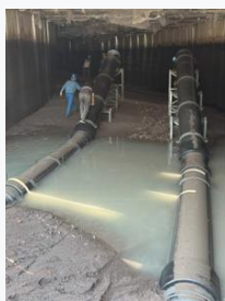
Sluicer pipes maintain intake clean
