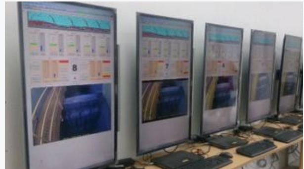
Control room for SediCon sediment removal system
