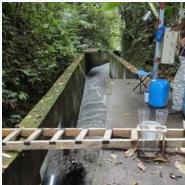
Monitoring equipment installed at discharge location
