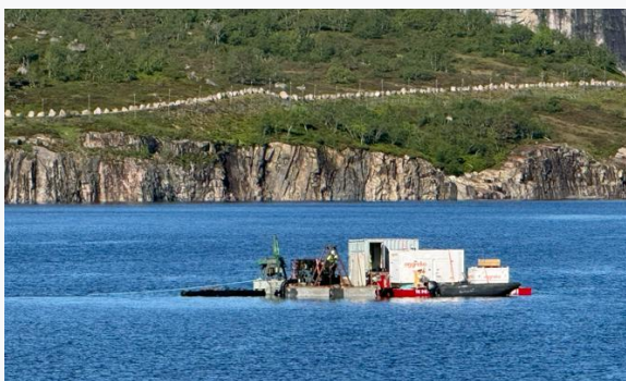
Surface setup with pump system installed on floating platform
