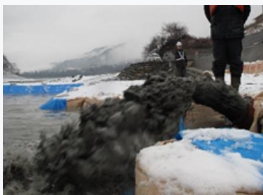
Sediment discharge during testing
