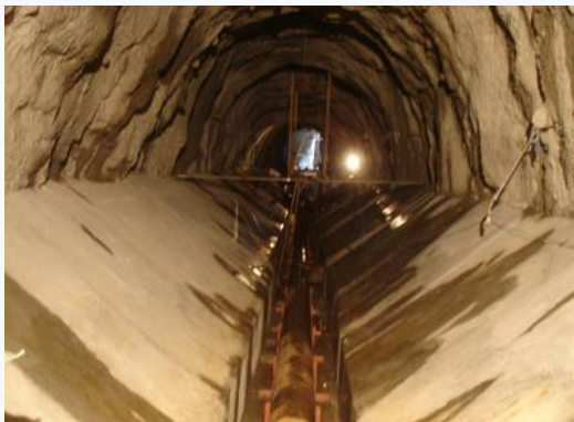
SediCon Sluicer installed in the desander
