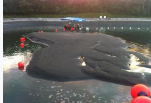
Sediment accumulation prior to dredging
