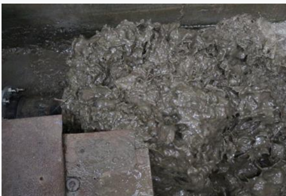
Sediment discharge during operation
