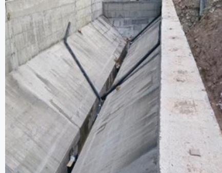
SediCon Sluicers installed in the desander
