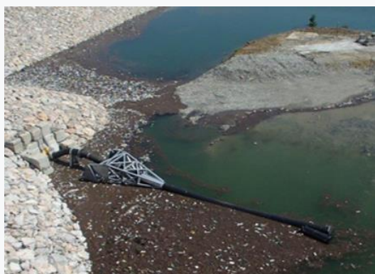
Reservoir connection for future SediCon HydroSuction Dredge
