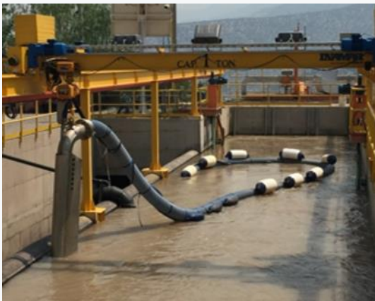
SediCon Desander Dredge installed in the forebay
