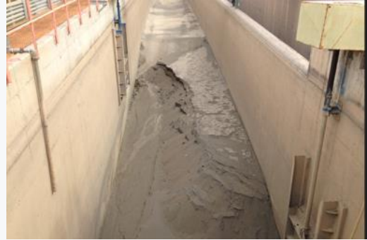
Sediment accumulation in the forebay prior to installation
