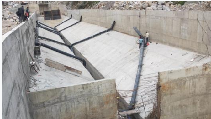
Three SediCon Sluicers integrated into the desander design
