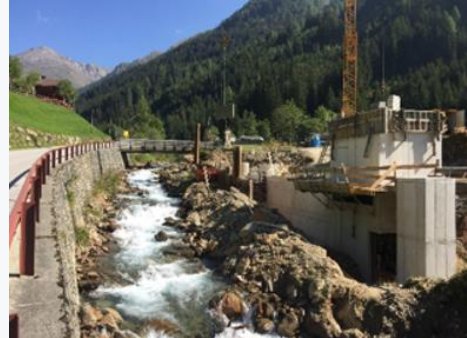
Winkeltal run-of-river hydropower plant
