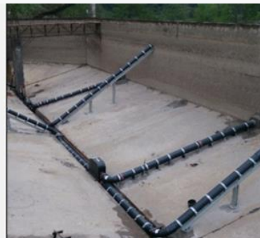
Two SediCon Sluicers installed in the desilting tanks
