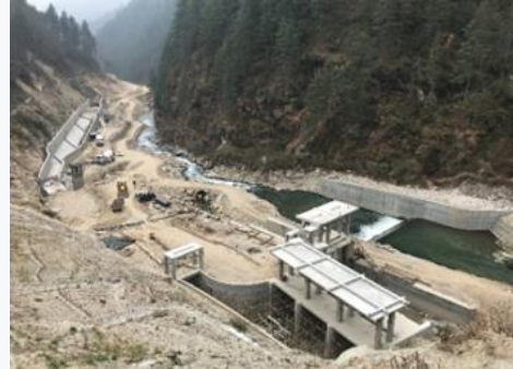
Upper Solu Headworks
