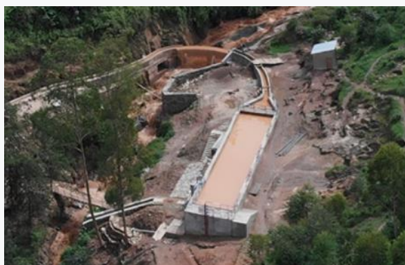
Desander and secondary intake
