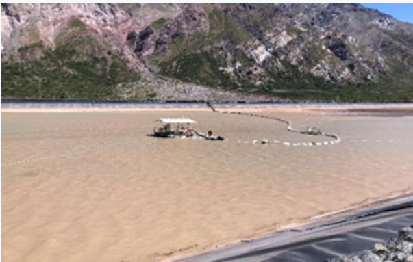
SediCon HydroSuction Dredge installed in Tinguiririca reservoir
