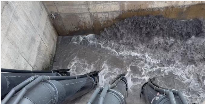
SediCon Sluicers removing sediment during plant operation
