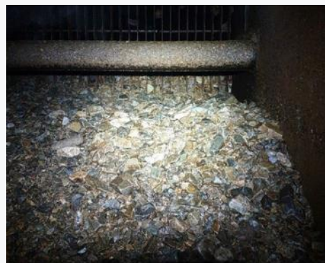
Accumulated gravel and stones at the intake trash rack, highlighting the need for underwater sediment removal
