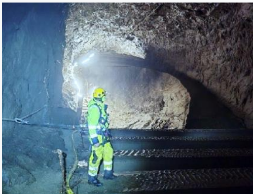
Svartisen sand trap during emptying in 2025. Sediment deposits have accumulated to approximately 8 m above the sand trap floor.
