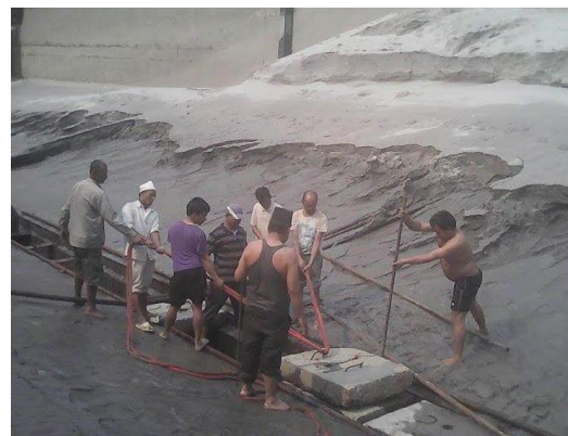
b) Inefficient flushing system (Source: NHPC)
