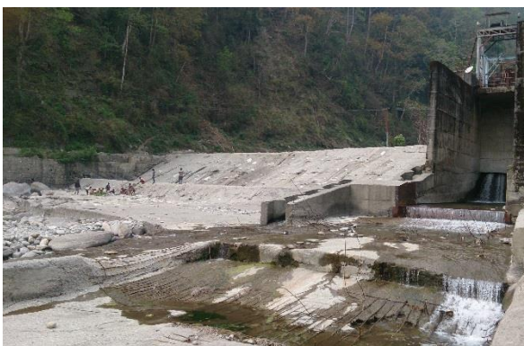
c) Scouring at Indrawati III headworks
